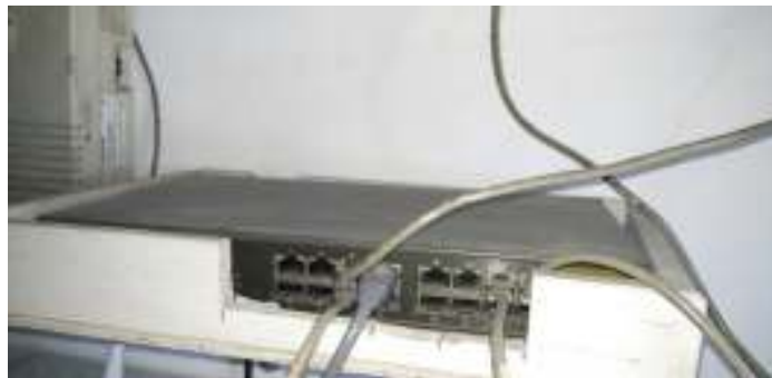
Gambar 3.5 Switch PT Total Printing Indonesia
