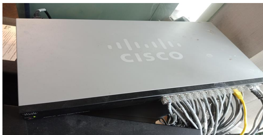
Gambar 3. 6 Switch Cisco SG220-26-K9-EU (26 port) Sumber: Kantor Notaris Soehendro Gautama, SH, M.Hum
