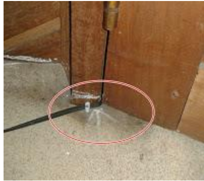
Gambar 2. 15 Kabel Fiber optic Tertimpa/tertindih Sumber : Data Penelitian (2021)
