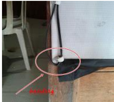
Gambar 2. 14 Fiber optic Bending Sumber : Data Penelitian (2021)
